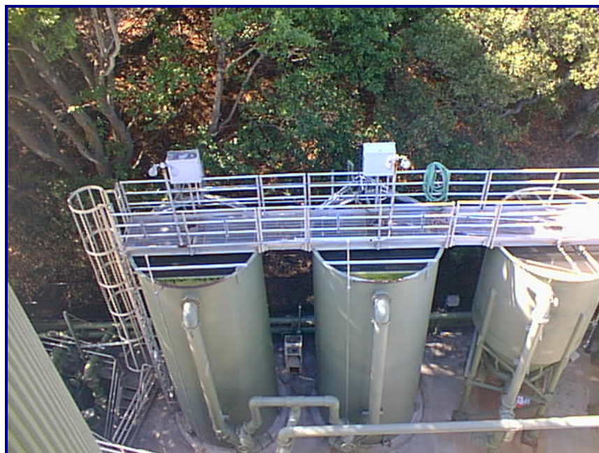
Figure 1: Existing Sand Media Filters at SMCSD
