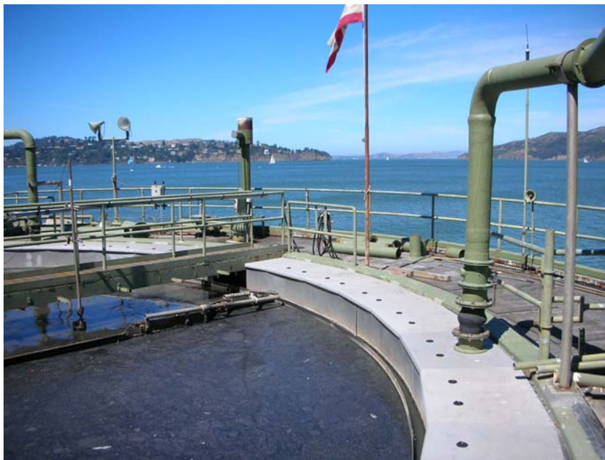
Figure 4 – Primary Clarifier Launder Cover
