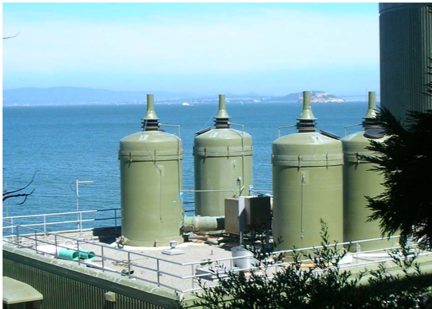
Figure 7 – Completed Odor Control System Installation
